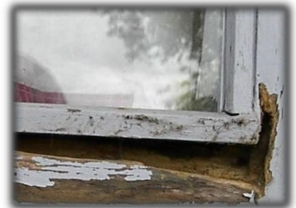
Rotting Wood Window
